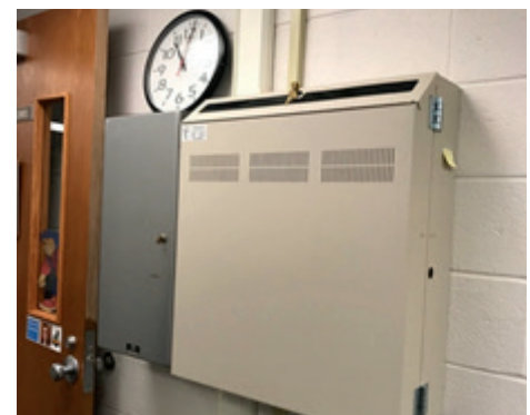
(Photos show the size of the equipment rack removed from Central Elementary that was replaced with the slim wall mount cabinet)
